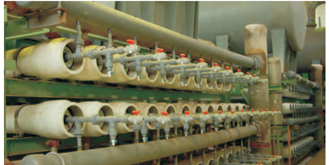
Reverse osmosis plant
